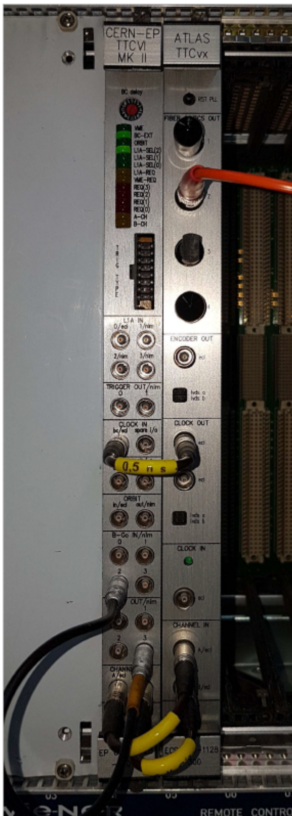
Figure 32. Image of cabled TTC system with B-channel connections
