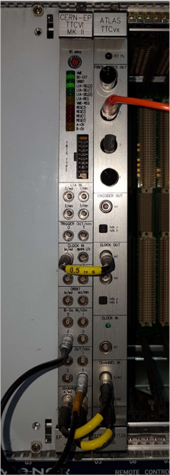
Figure A.2 Image of cabled TTC system with B-channel connections
