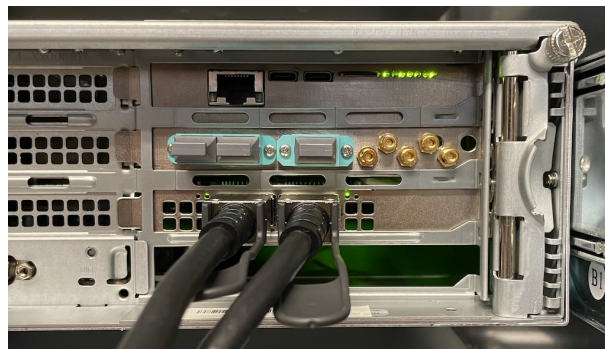
Figure 3.25: FLX-182 (revision 1.0) installed in a Supermicro H12 server, above a 200 GbE Nvidia Connect-X6 network card.
